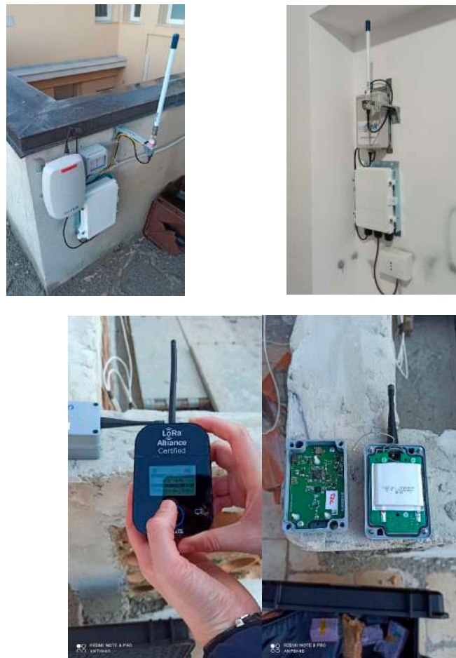
Figure 12. The installed gateway
