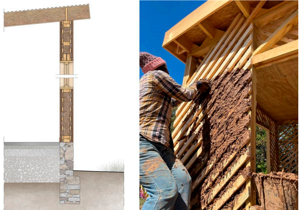
Figure 4. Building section and construction step where the wooden framework is manually filled with light earth.
