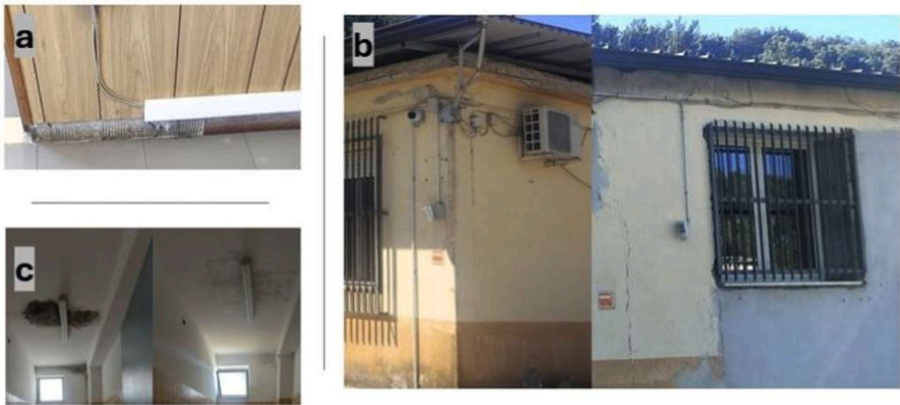
Fig. 11. Photos display some weaknesses in the administration adaptive reused section: a) ceramic and timber finishes superposed on the internal walls, b) scraps on the external walls, c) Humidity in the roof before and after corrections.
