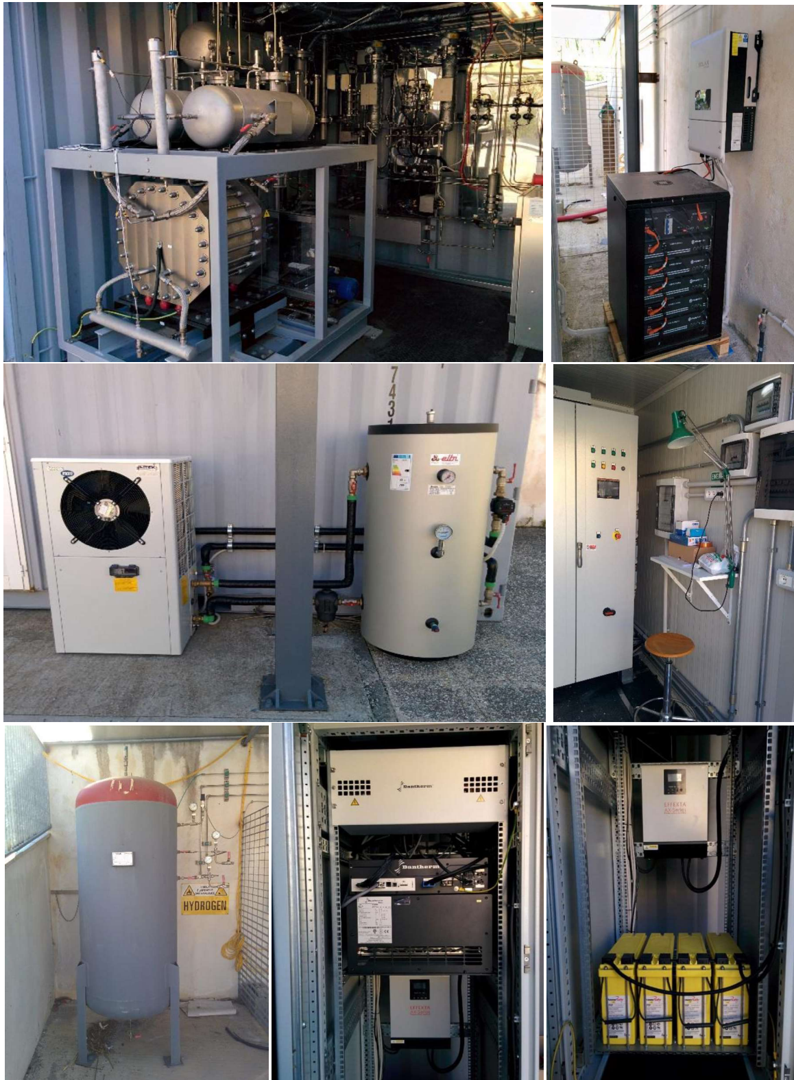
Figure 2 – Components of the system (electrolyser, inverter and batteries for PV production, chiller, controller, tank, fuel cells, inverter and batteries for fuel cell production)
