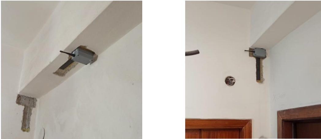
Figure 7. The multi sensor nodes installed.
