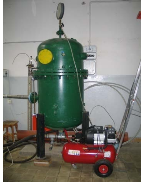
Figure 25 Pressure increasing station with the compressor.
