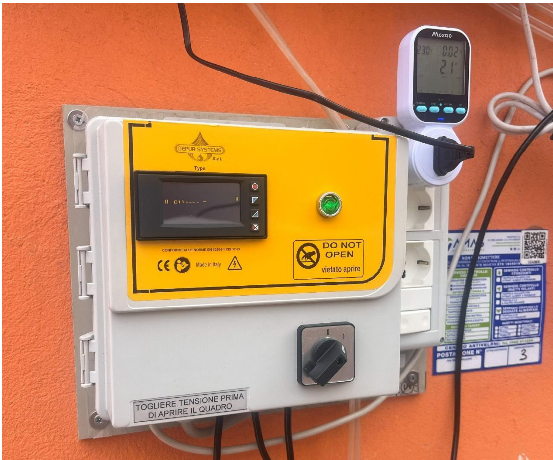
Figure 6.2 - Final operative configuration of the automated aeration system
