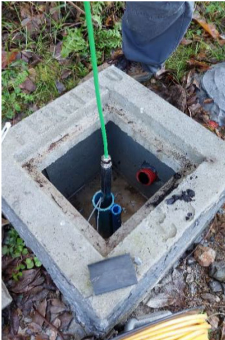
Fig. 12 Piezometer installed in Monitoring Station N. 2
