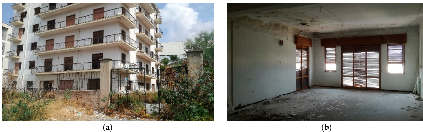
Figure 4. State of the case study RC building: (a) external view and (b) example of internal view.
