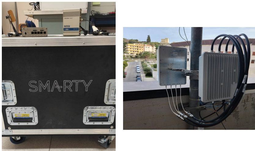
Fig. 3.11: 5G deployment in the campus: gNB, core network and edge server (left) and antenna (right).
