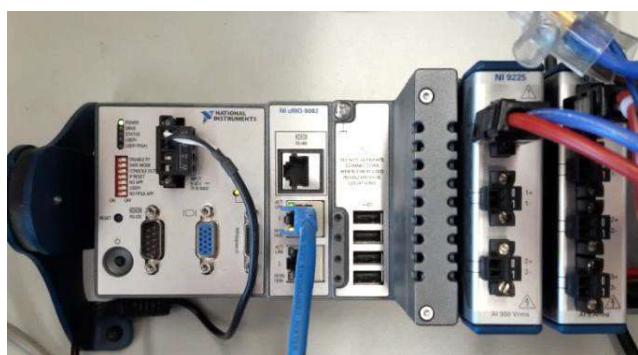
Fig. 4. Second smart meter (funded by PON Project “DOMUS Energia”).
