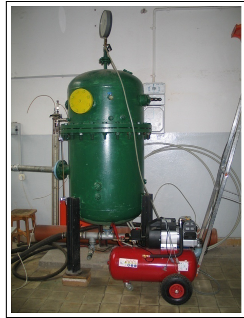
Figure 3. Pressure increasing station with the compressor.
