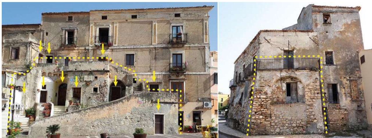
Fig. 4.18 – Two examples of gafio in San Lucido. On the left, a complex one of landing-type with a long staircase serving ten different openings; on the right, a small one of loggia-type. Photos by Guglielmo Minervino
