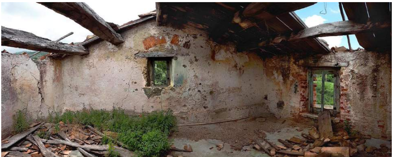
Fig. A1.5 – An example of a wooden roof and window lintels in a XVIII century house, in Paola. Photos by Guglielmo Minervino.
