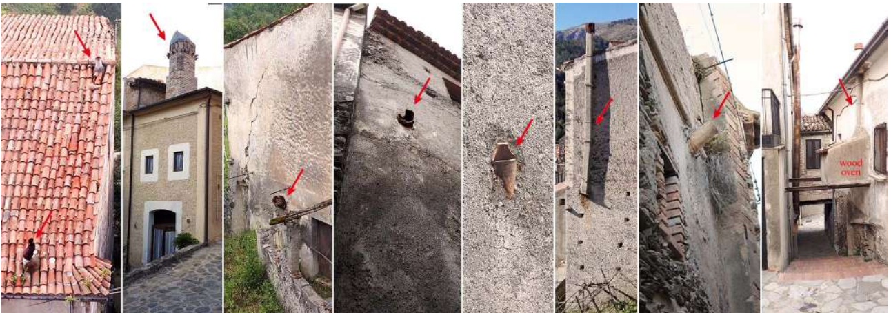
Fig. 4.26 – Various types of chimney from Calabrian historical towns. Photos by Guglielmo Minervino
