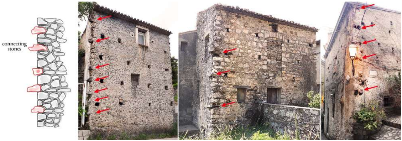
Fig. 4.21 – Set-up for wall connections in Aieta, San Donato di Ninea, and Scalea. The wall section on the left shows the location of connecting stones that are put on the corner of buildings. They indicate where other buildings are allowed to be built in adherence. Red arrows indicate connecting stones in the three different situations. Photos by Guglielmo Minervino
