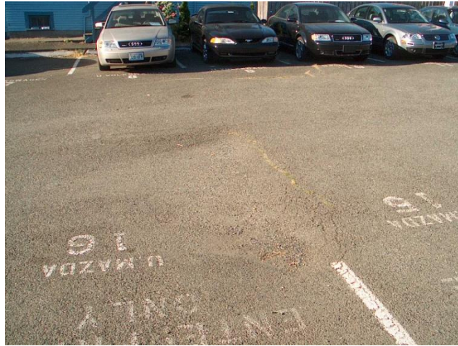
Figure 1.11 Depressions in asphalt layer
