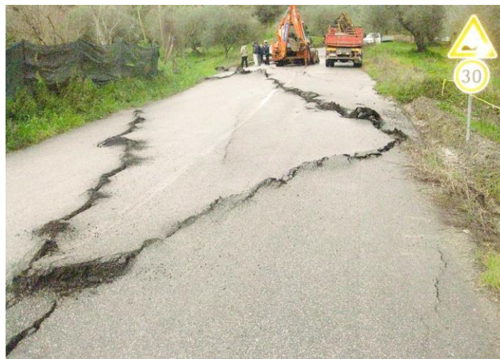
Fig.4.12 a) 9.47am: cuts on the road S.P. 55 Filogaso-Maierato (Draga locality)
