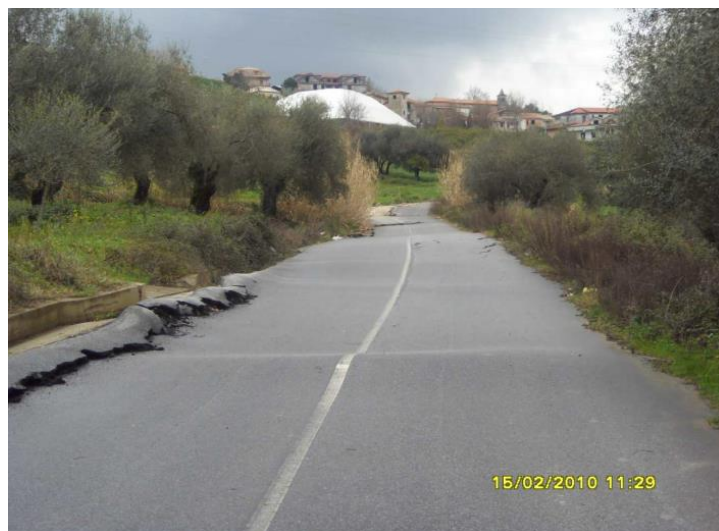
Fig.4.12 b) 11.29am: deformations on the road S.P. 55 Filogaso-Maierato (Bosco locality)
