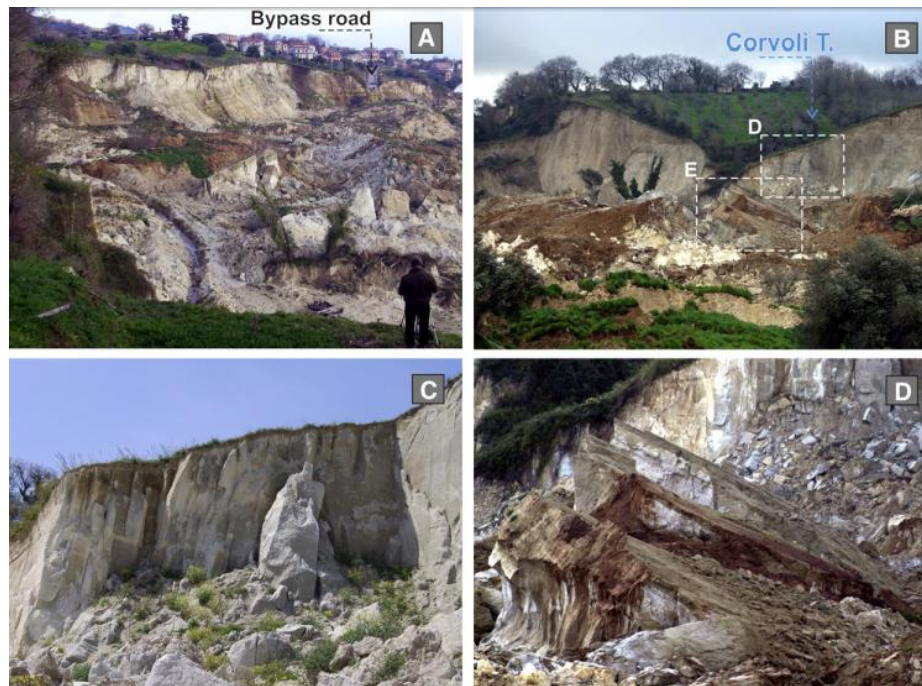
Fig.4.15a-d - Upper sector: (A) Main scarp (~600 m) that extends from NE to SW, making a gentle curve; (B) valley of the Corvoli Torrent that split the main scarp into two parts; (C) band of parallel joints (~15 m wide), NE–SW trending, related to the decompression that occurred during landslide movement along the main scarp; (D) large rock blocks rotated backward.
