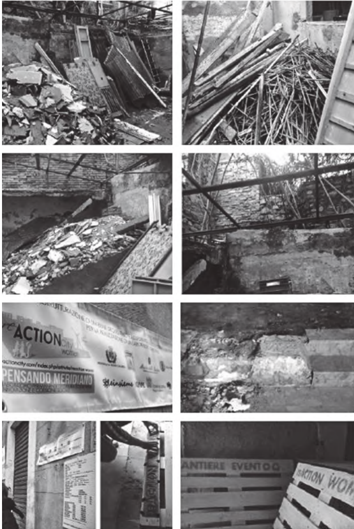
SelfBuild_ReAction City woman The existing building -Step of the re-building [Ph: G.Mangano]
