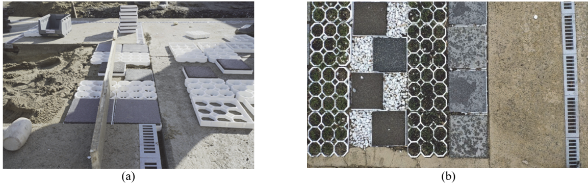
Fig. 7. Area Testing Scenario 3 (PMopenlab, R.ed.el Lab., 2018, Reggio Cal., Italy) (a) represent the implementation of recycled and printed components, (b) the final construction already in function of the green parking unit.
