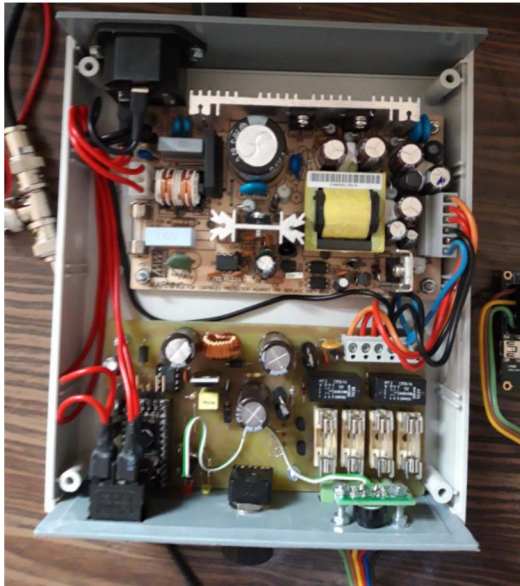
Fig. 10. Inside the casing with the pulser board power supply.
