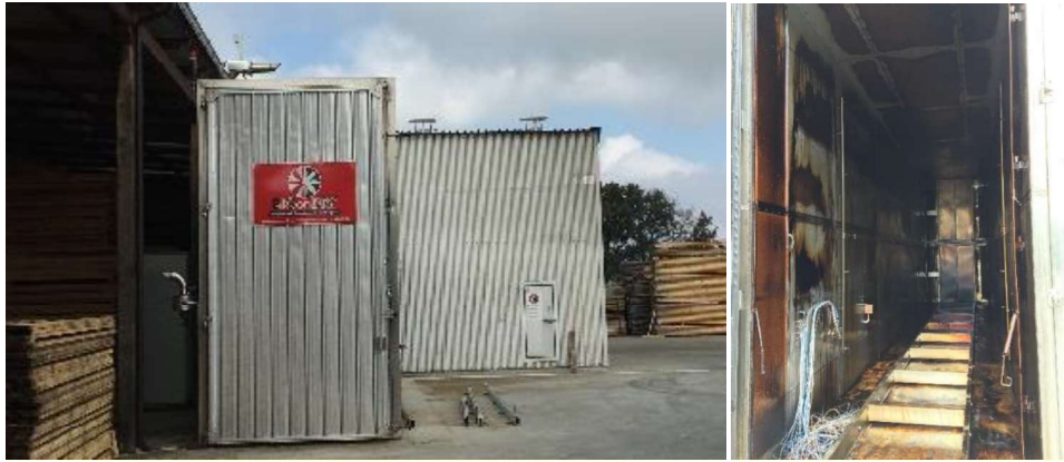
Figure 1 - Exterior (on the left) and interior (on the right) of the THW 20.95.41 heat-treatment plant.
