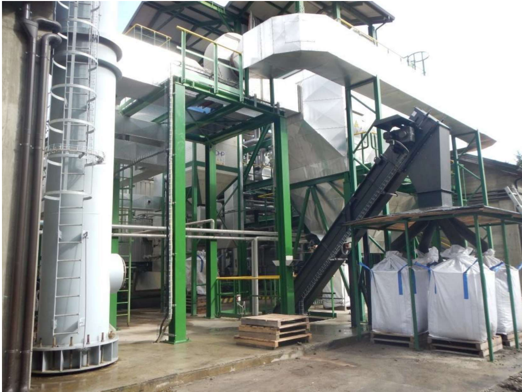
Figure 2 - Thermoelectric power plant.
